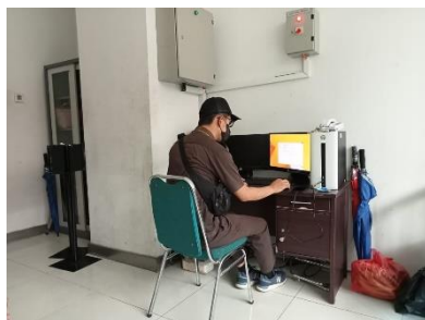
Sistem CPA (Central Plan Automation) Chiller Gedung IMERI
