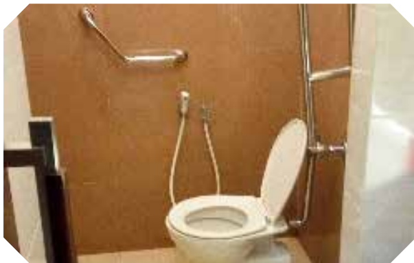
Autoflush toilet untuk difabel di Fakultas Teknik UI. Autoflush toilet for disabled at the UI Faculty of Engineering.
