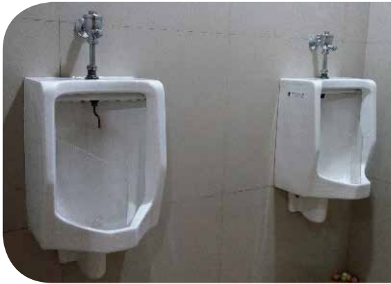
Urinoir flushing system
