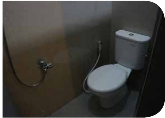
Toilet flushing system
