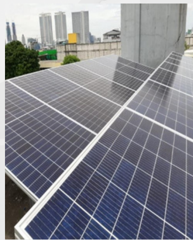
Picture: Solar panels
