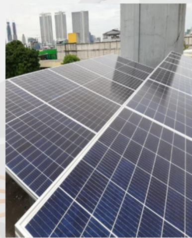
Picture: Solar panels
