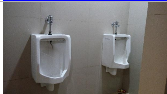
Urinoir flushing system
