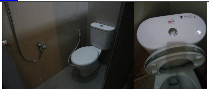
Toilet flushing system
