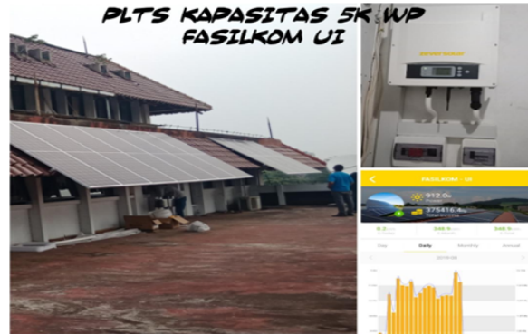
Solar Power Plant of Second Building Faculty of Computer Science
