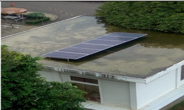
Solar Power Plant of X Building Faculty of Humanities
