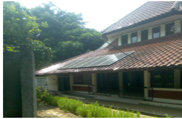
Solar Power Plant of Prayer Room Faculty of Humanities
