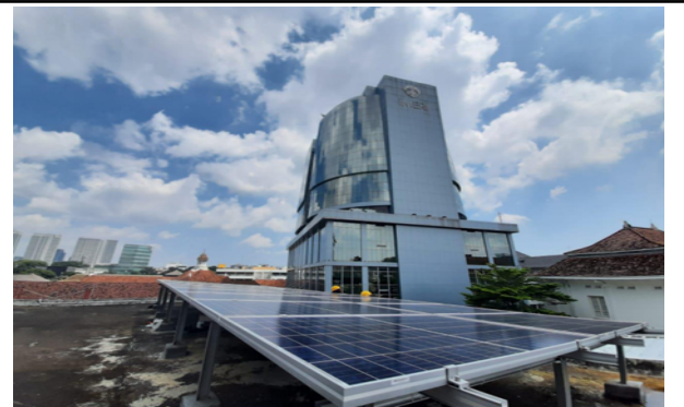
Solar Power Plant of Utility Building Faculty of Medicine
