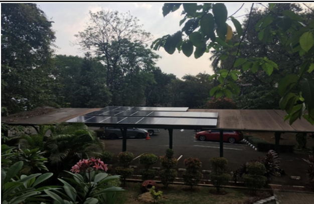
Solar Power Plant of Parking Area Faculty of Public Health
