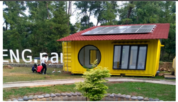
Solar Power Plant of Engineering Park Faculty of Engineering
