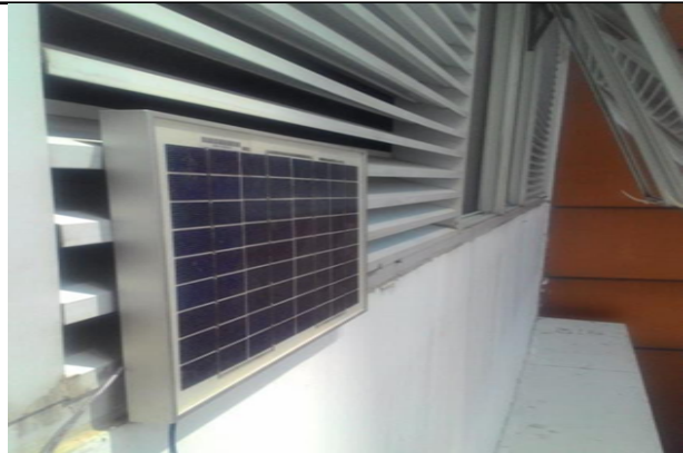
Solar Power Plant Faculty of Nursing
