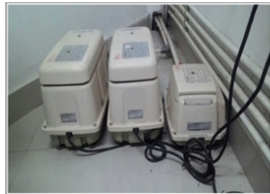
Wastewater/sewage treatment equipment
