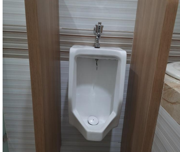
Toilet and Urinal with Flush System Administrative Center of UI
