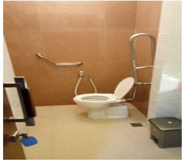
Toilet and Urinal with Flush System Faculty of Engineering (FT)
