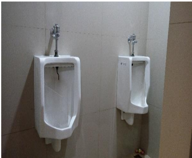
Toilet and Urinal with Flush System Faculty of Engineering (FT)
