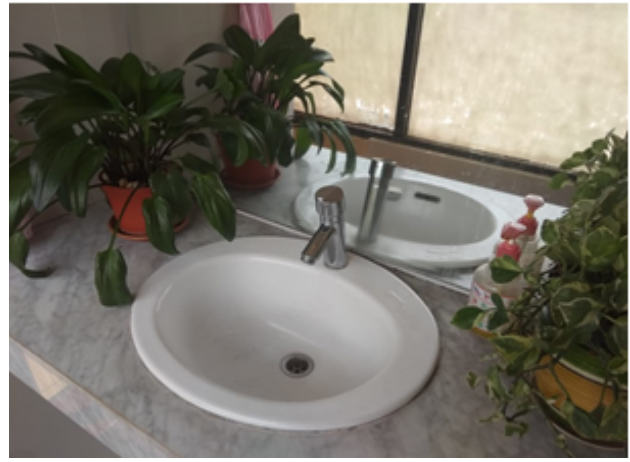
Water Tap with Sensor System Administrative Center of UI
