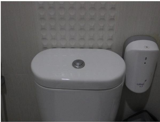
Toilet and Urinal with Flush System Faculty of Law (FH)
