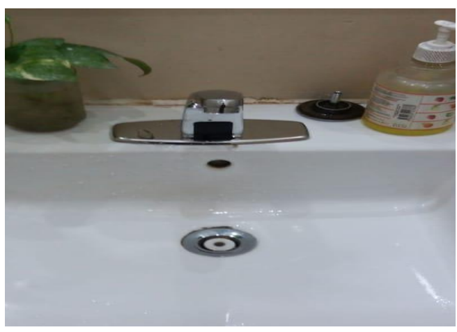
Water Tap with Sensor System Faculty of Social and Political Science (FISIP)
