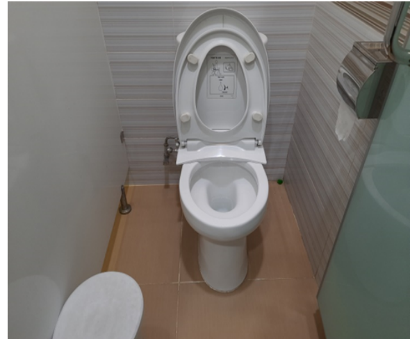
Toilet and Urinal with Flush System Faculty of Social and Political Science (FISIP)
