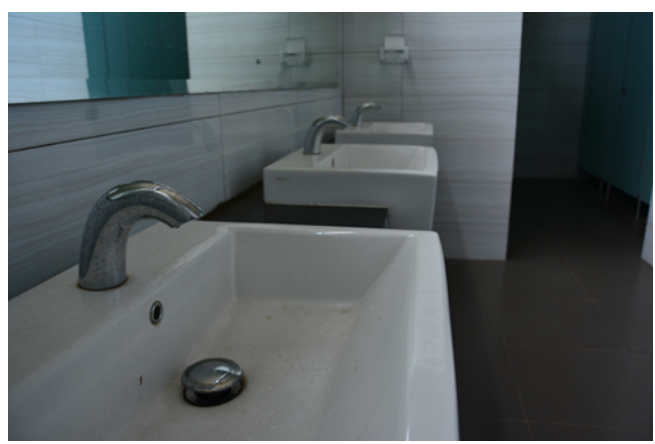
Water Tap with Sensor System UI Hospital (RSUI)
