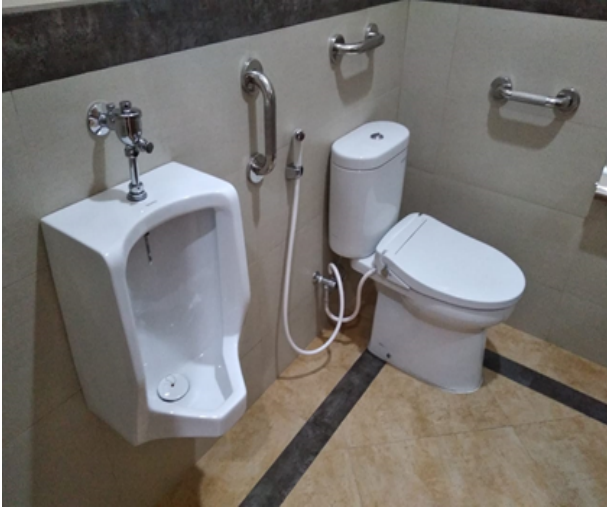
Toilet and Urinal with Flush System Faculty of Public Health (FKM)
