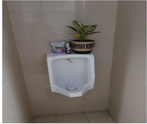
Toilet and Urinal with Flush System Faculty of Administrative Science (FIA)
