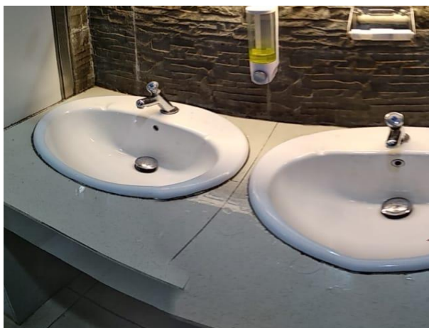
Water Tap with Sensor System Faculty of Public Health (FKM)
